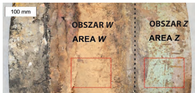
Fig 2. General view of the fragment of the tested steel pipeline with the indication of the areas subject to further analysis
