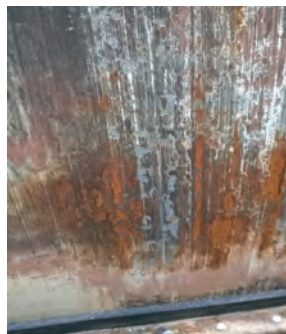
Photo 1. Unevenness and damage of coatings and pitting corrosion
