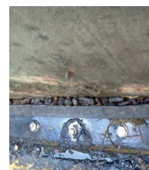
Photo 4. A crevice filled with stones
