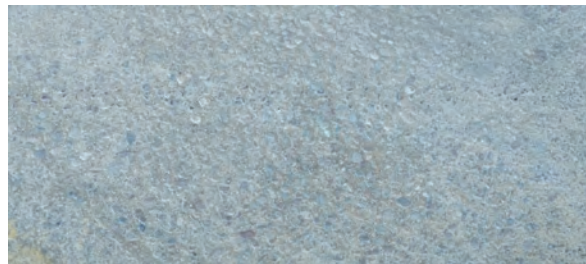
Photo 9. Effects of marine environment on elements of reinforced concrete hydrotechnical structures operating in a marine environment: a) exposure of diffuse reinforcement, b) exposure of the aggregate structure
