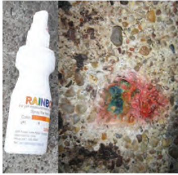
Photo 11. One of the test locations used to determine the concrete reaction at the measurement site
