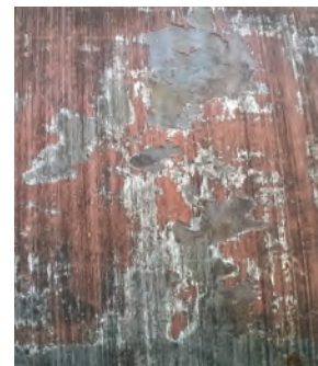
Photo 2. Local detachment of coatings
