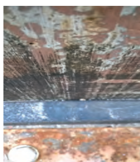
Photo 3. Leaky connection of the seal with the wall
